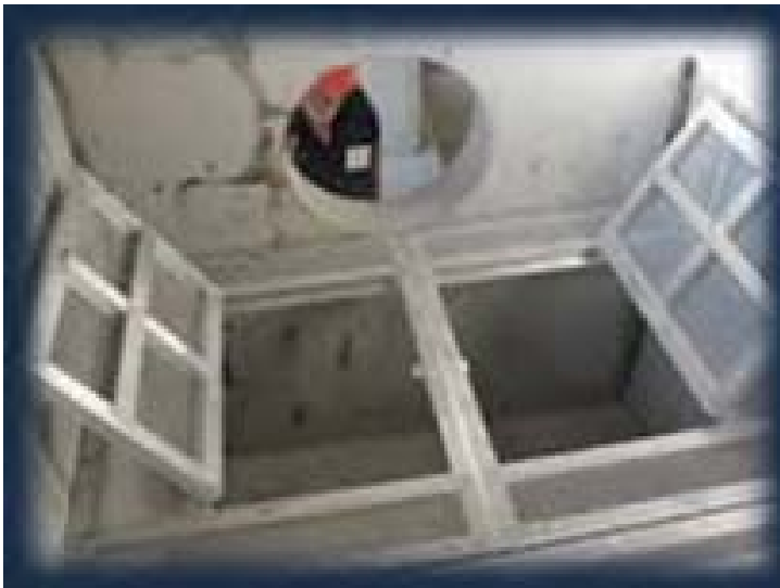
c. Bottom screens opened for cleaning
