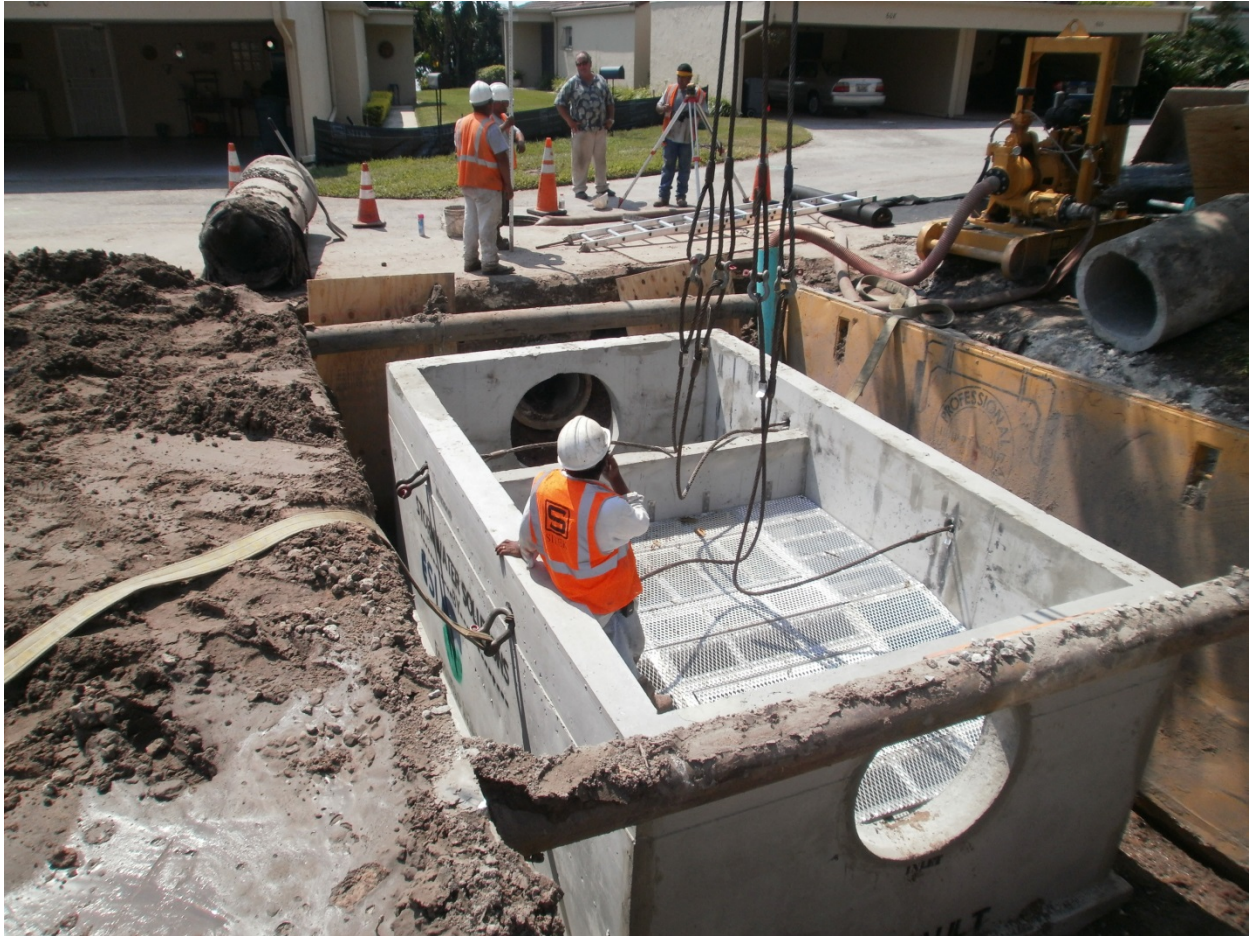
Installation of one of the smaller baffle boxes at the Sausalito Condos on Lake Howell. This box treats a 24" storm pipe – the upstream side is in the foreground (Lake Howell is just beyond the buildings in the photo.) The leaf screen can be seen on the upstream side of the box.
