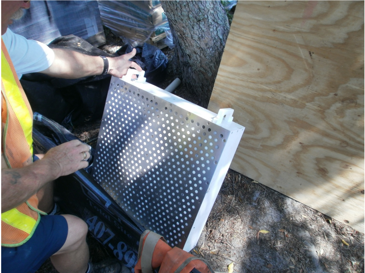
Cassette media filter prior to installation in one of the baffle boxes at Sausalito Condos on Lake Howell. These filters typically require annual replacement.
