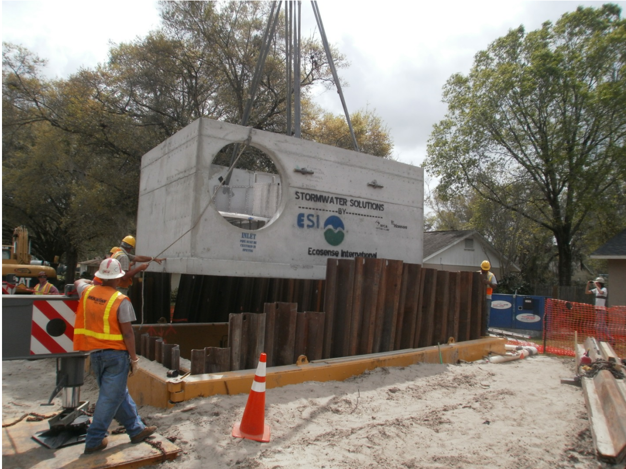
Lowering of one of the larger baffle boxes via crane on Osceola Trail at Gee Creek. Note the temporary sheet pile installation around the excavated area. The large opening in the side of the box is where the 42" upstream pipe was set (see next photo). Gee Creek (receiving water) is behind the homes to the right in the photo.
