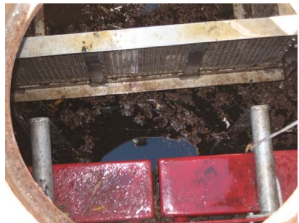
d. Baffle box unit following cleaning
