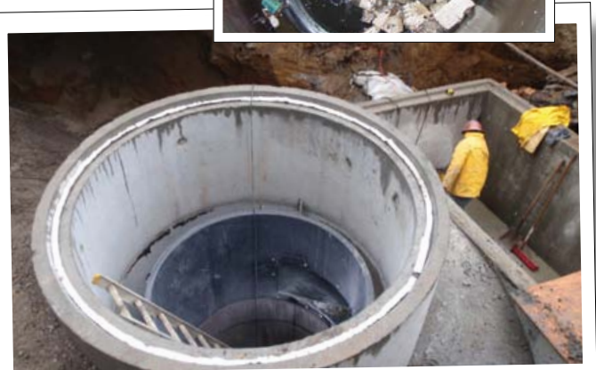
CDS unit installed to remove trash before entering Lake Meritt in Oakland, CA
