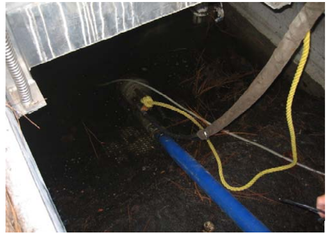
b. Standing water is pumped from the sump area
