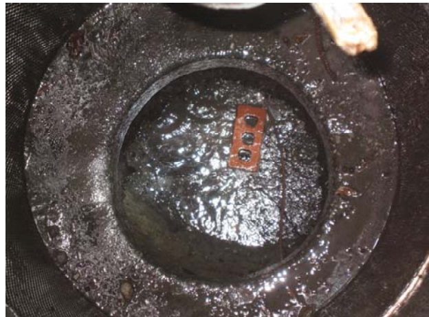
d. Sump area of CDS unit following cleaning
