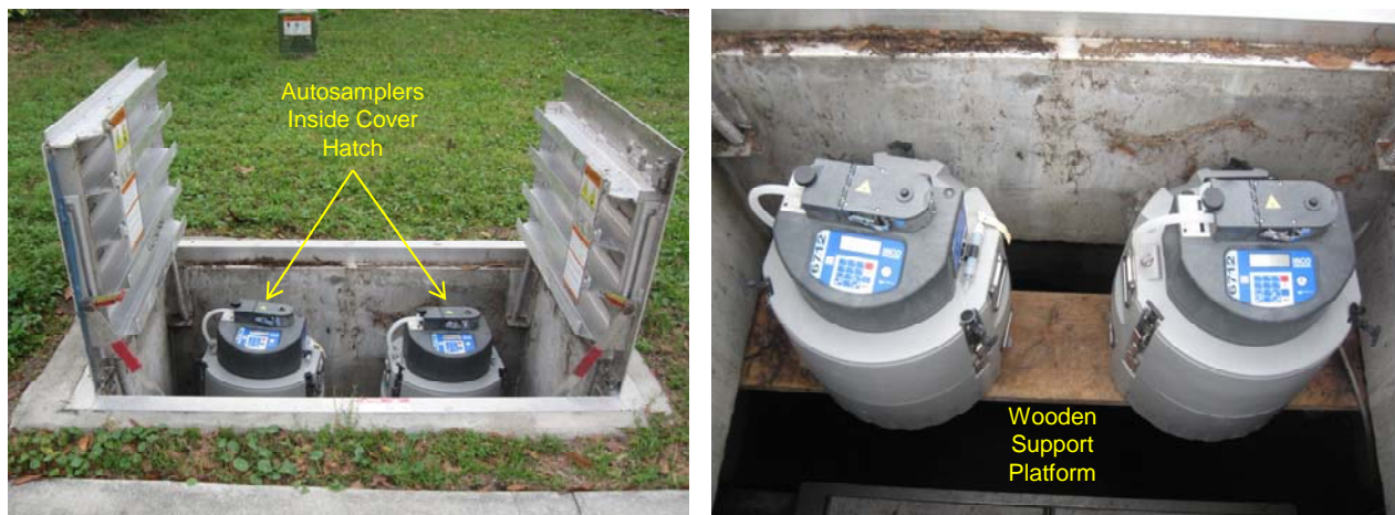
Figure 3-3. Overview of Sampling Equipment Installed at the Gee Creek Site.
