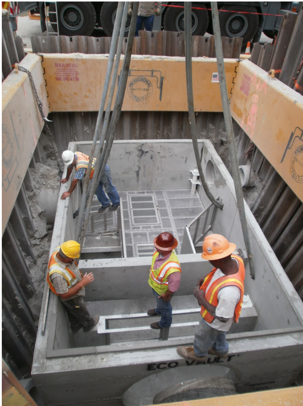
Placement of the baffle box on Osceola Trail at Gee Creek. Due to existing pipe geometry, this box was configured in a “T” fashion, receiving flows from a 42” pipe (upper left) and 15” pipe (upper right) with outflow to a 42” pipe (foreground) that discharges to Gee Creek. The leaf screen can be seen in the background. A PVC tube where VaultOx® is placed is visible in the upper right corner of the box. The metal frame in the foreground is where the cassette media filters are placed (this box requires two cassettes).
