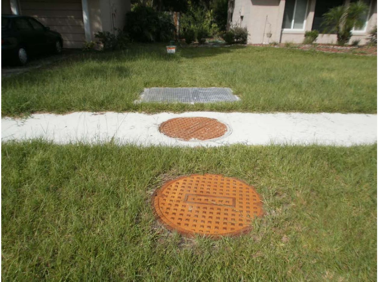
Baffle box on Osceola Trail at Gee Creek after full restoration. Gee Creek is behind the homes in the background. The manholes and hatches are used to access the baffle box for maintenance, including cleanouts and filter replacement.
