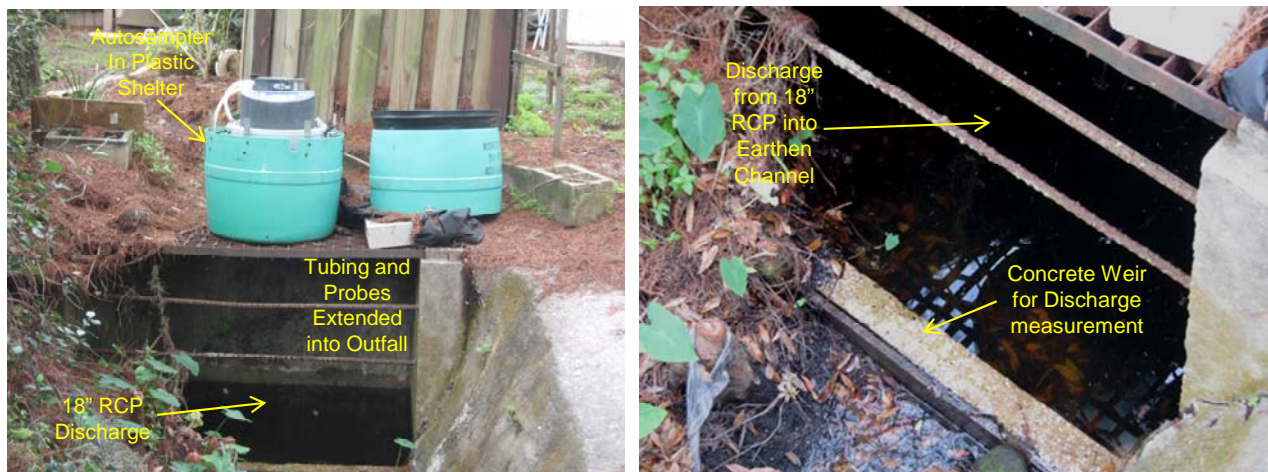
Figure 3-6. Photographs of the Sampling Equipment Used at the San Pablo CDS Unit Site.
