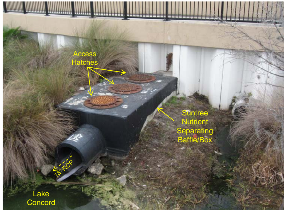
Figure 2-26. Photograph of the Outside of the Lake Concord Baffle Box Site.
